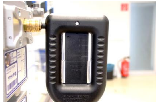
Figure 165: U-tube manometer on inspection cover
